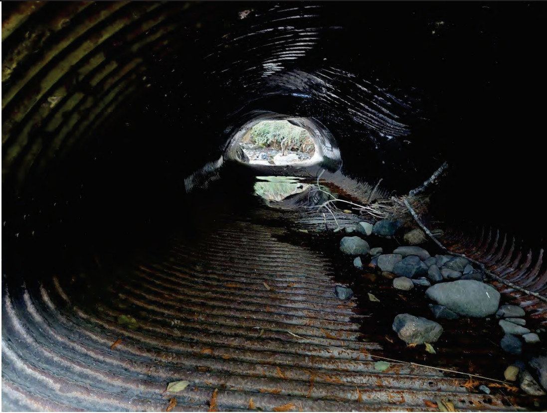
Culvert Interior facing DS: Buckling visible at 2 o'clock, flowing water visible in the middle of the culvert
