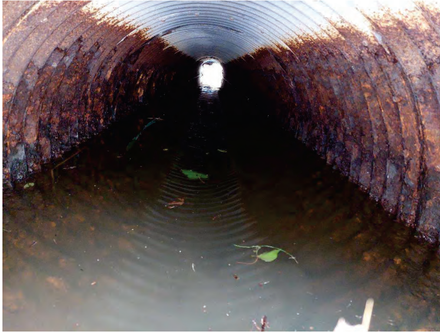
Pipe Interior (eastern pipe) facing US: Signs of significant corrosion with loss of material visible, 2 to 11 o'clock
