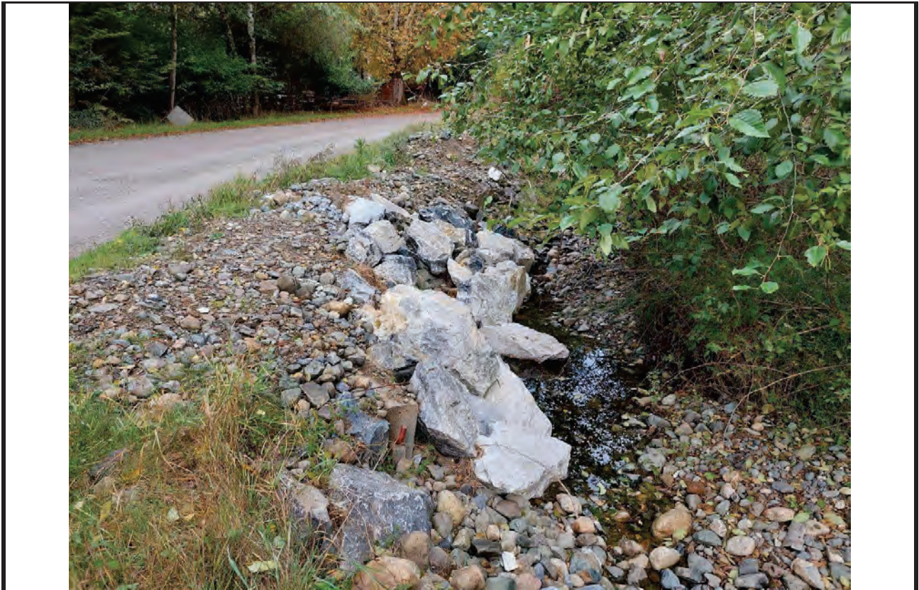
Upstream Channel at Bell Rd: Undermining of embankment along 14m stretch, dumped riprap visible
