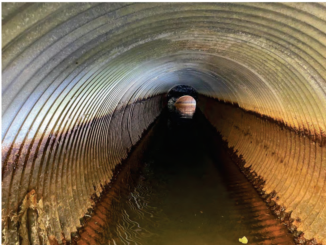
Pipe Interior facing DS: Pipe joint separation visible with skewed outlet pipe and visible rock
