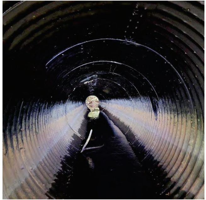
CULVERT 13 (3442926) INTERIOR: MINOR PIPE JOINT SEPARATION
