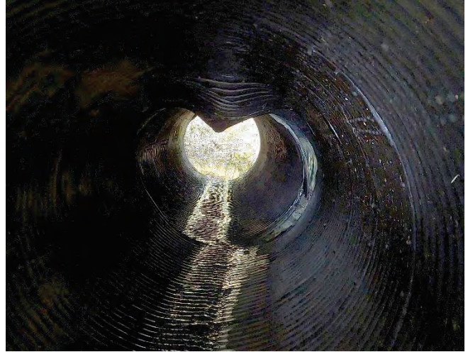
CULVERT 12 (2255061) INTERIOR: BUCKLING AND PIPE JOINT SEPARATION
