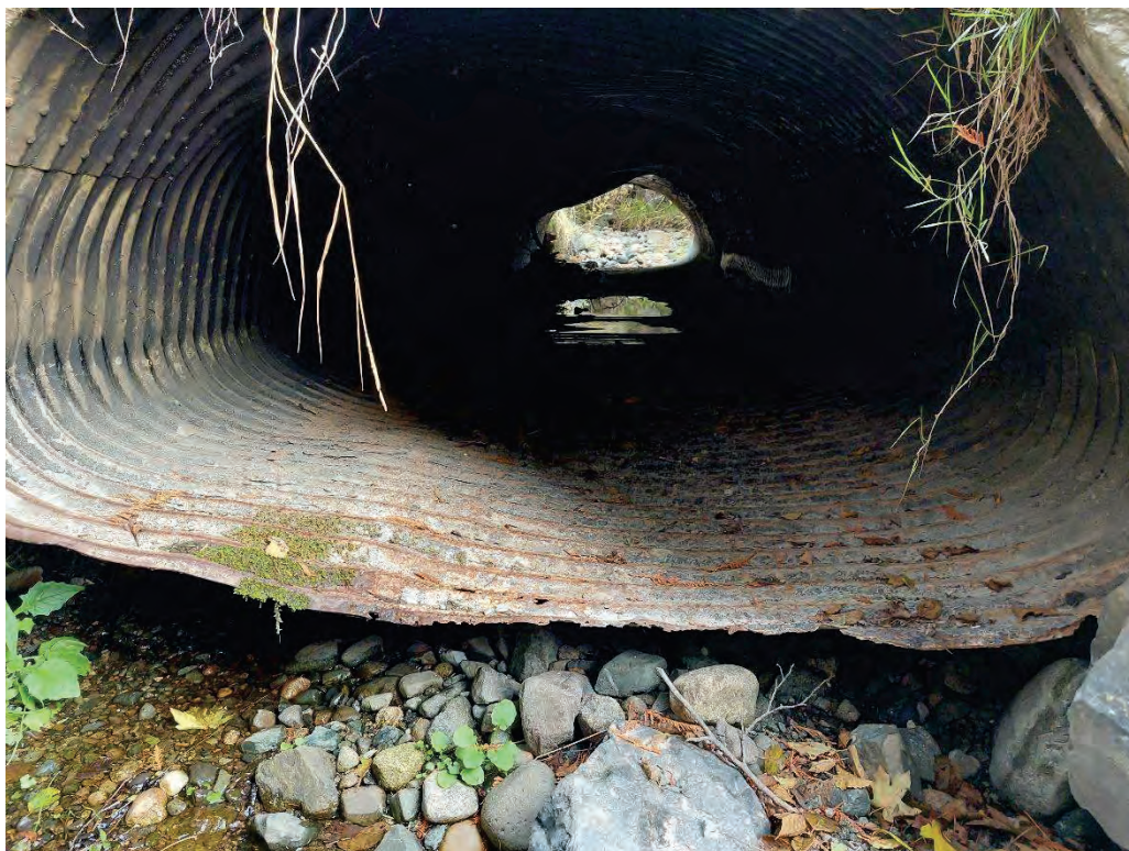
Culvert Outlet: Pipe invert heavily corroded, flow visible coming from under the culvert
