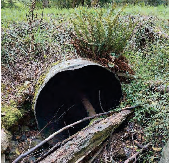
CULVERT 9 (2256424) INLET: WOODY DEBRIS AT INLET
