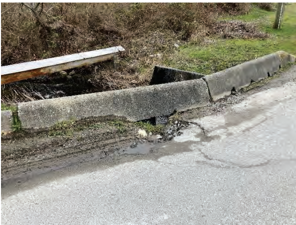
PHOTO 1: AREA 1 - ROAD EMBANKMENT FAILURE (MOTI, MARCH 2022)
