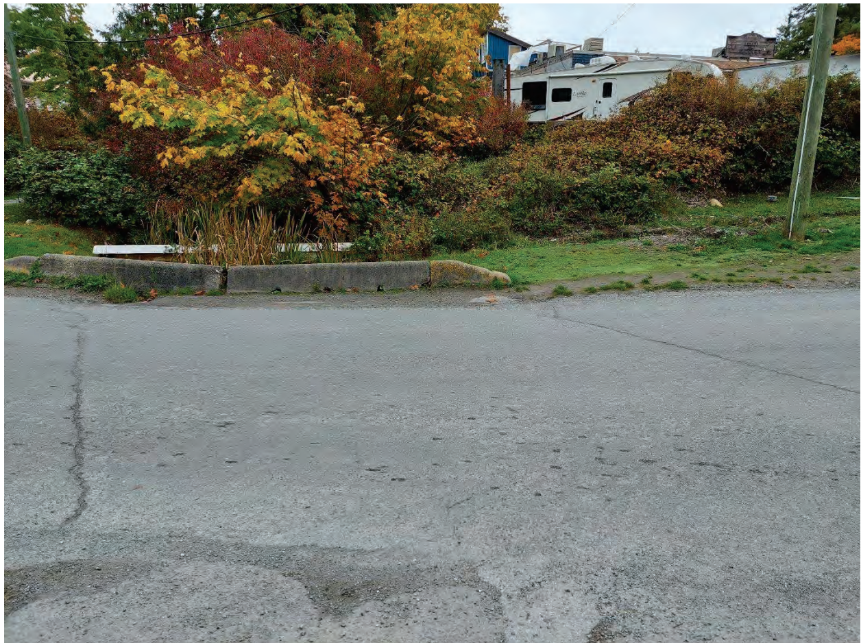
Pavement Surface: Tension cracks visible on the left and the right from the culvert crossing
