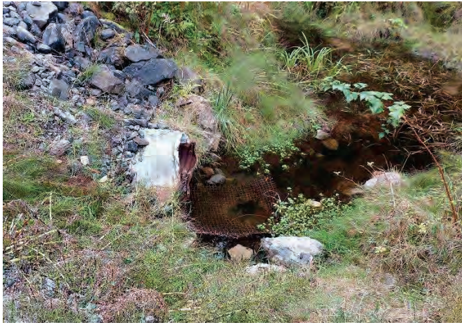
CULVERT 1 (2254949) INLET: DAMAGED INLET AND GRATE
