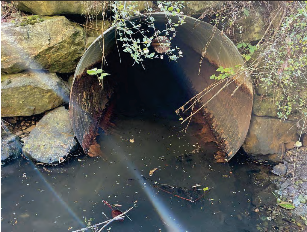
Culvert Inlet: Heavily corrosion at pipe invert with large section of missing material
