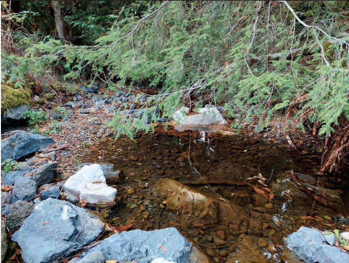
Downstream Channel facing DS: Downstream pool with erosion of banks on both sides
