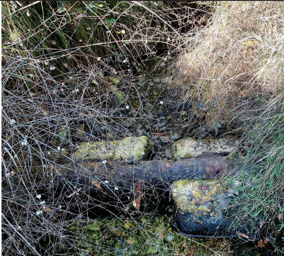
Upstream Channel facing US: DI utility service line visible in the upstream channel 3m from inlet
