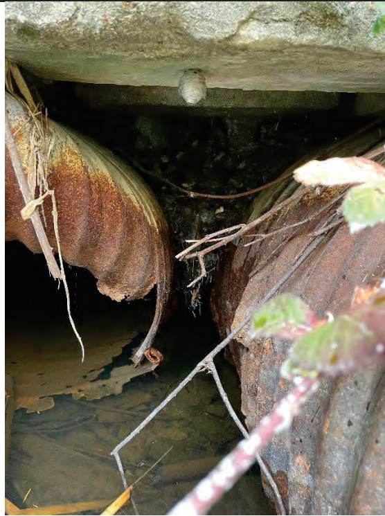
Culvert Inlet: CRB sitting on culverts, large cavity visible between twin pipes
