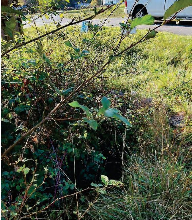
AREA 4 SANDERSON RD: OVERGROWN ROADSIDE DITCH
