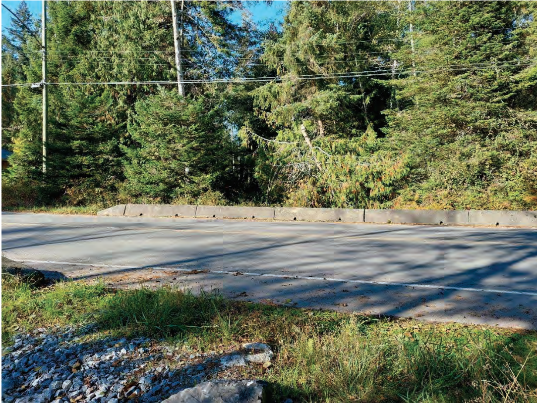
Pavement Surface: Gillies Bay Road above Cranby Creek Crossing
