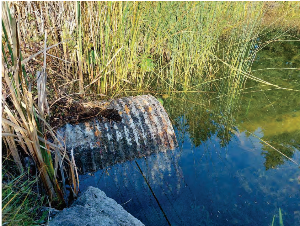
Culvert Outlet: Outlet about 75% submerged and visibly corroded on the outside
