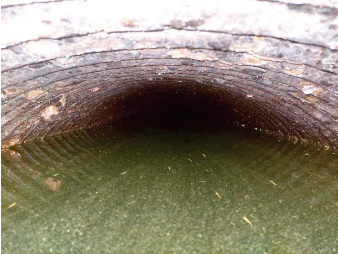
Pipe Interior facing US: Pipe lining visibly damaged with corrosion visible
