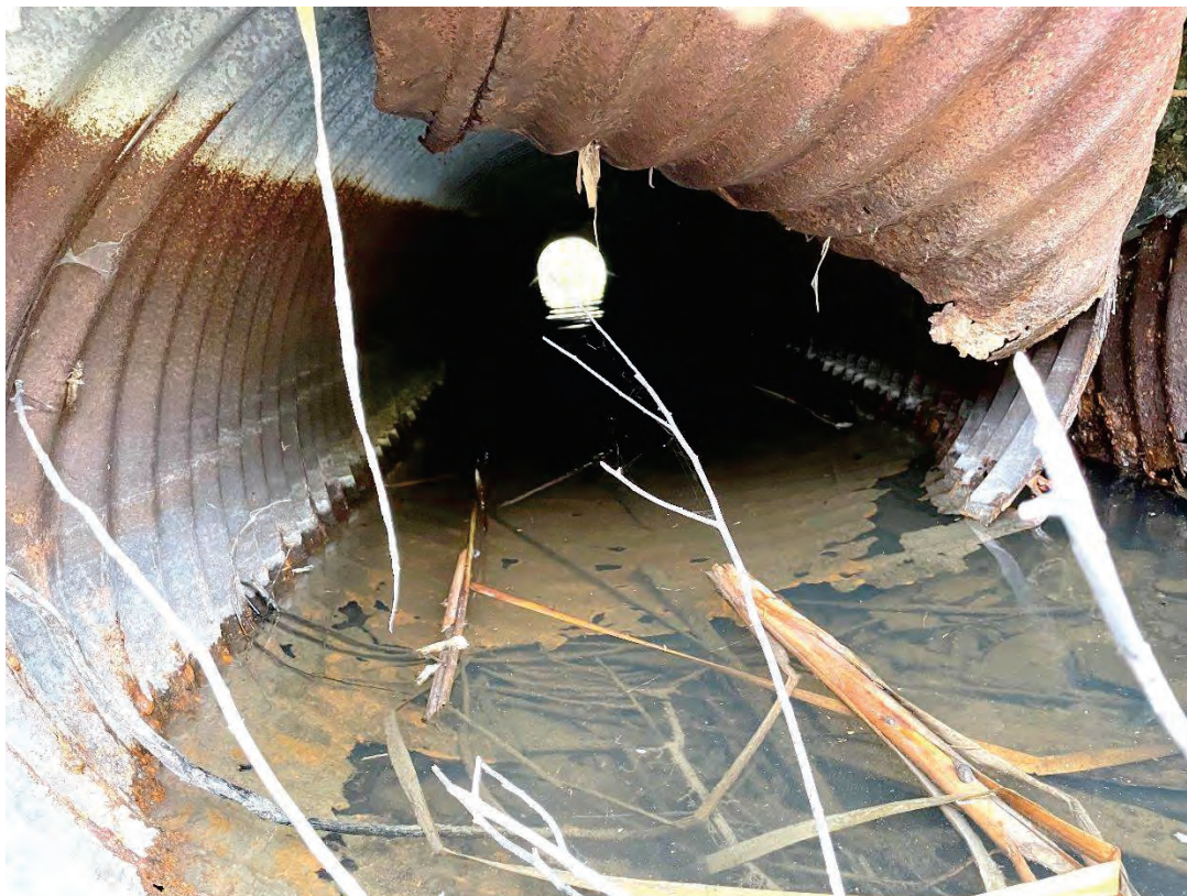
Pipe Interior (western pipe) facing DS: Visible damage of inlet and heavy corrosion of invert
