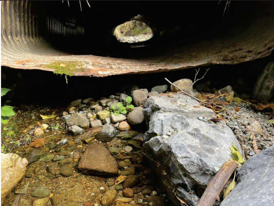
Culvert Outlet: Visible undermining of culvert pipe with visible stream flowing under pipe
