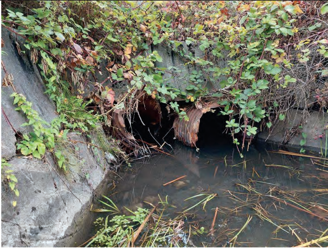
Culvert Inlet: Inlet damaged and corroded, CRB headwall & wingwalls
