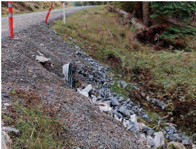
CULVERT 11 (2254788) OUTLET: ERODING ROAD EMBANKMENT AT OUTLET
