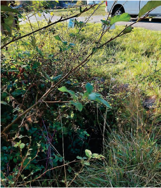
CULVERT 7 (2258625) OUTLET: OVERGROWN ROADSIDE DITCH
