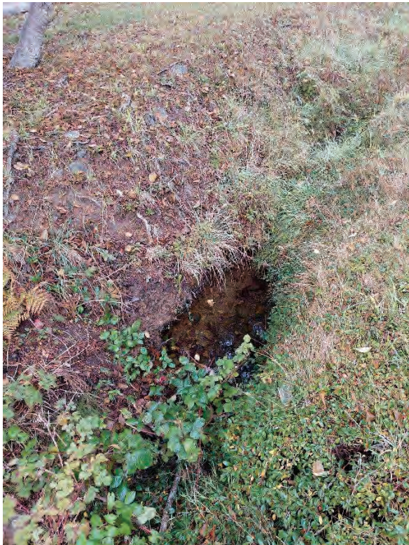
AREA 4 GILLIES BAY RD: BANK EROSION OF ROADSIDE DITCH
