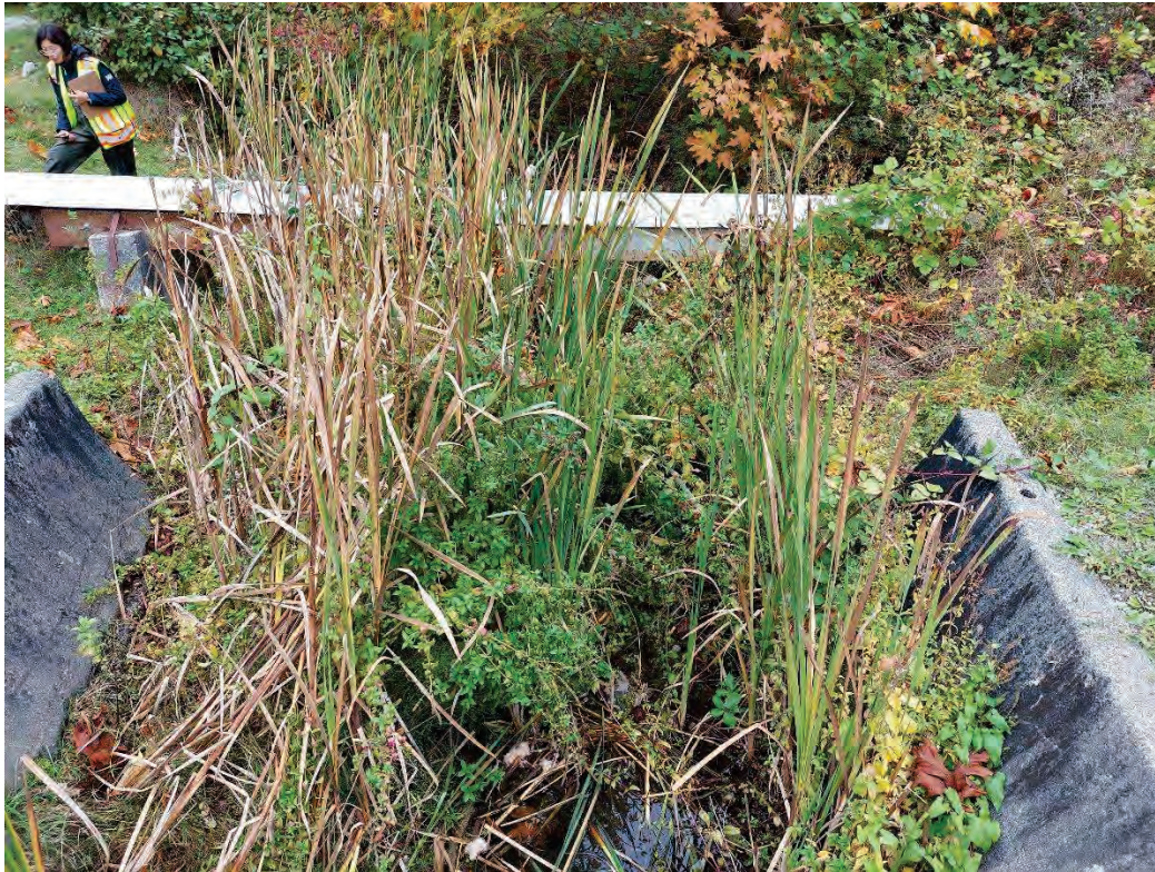
Downstream Channel facing DS: Sediment accumulation and vegetation visible & CRB wingwalls
