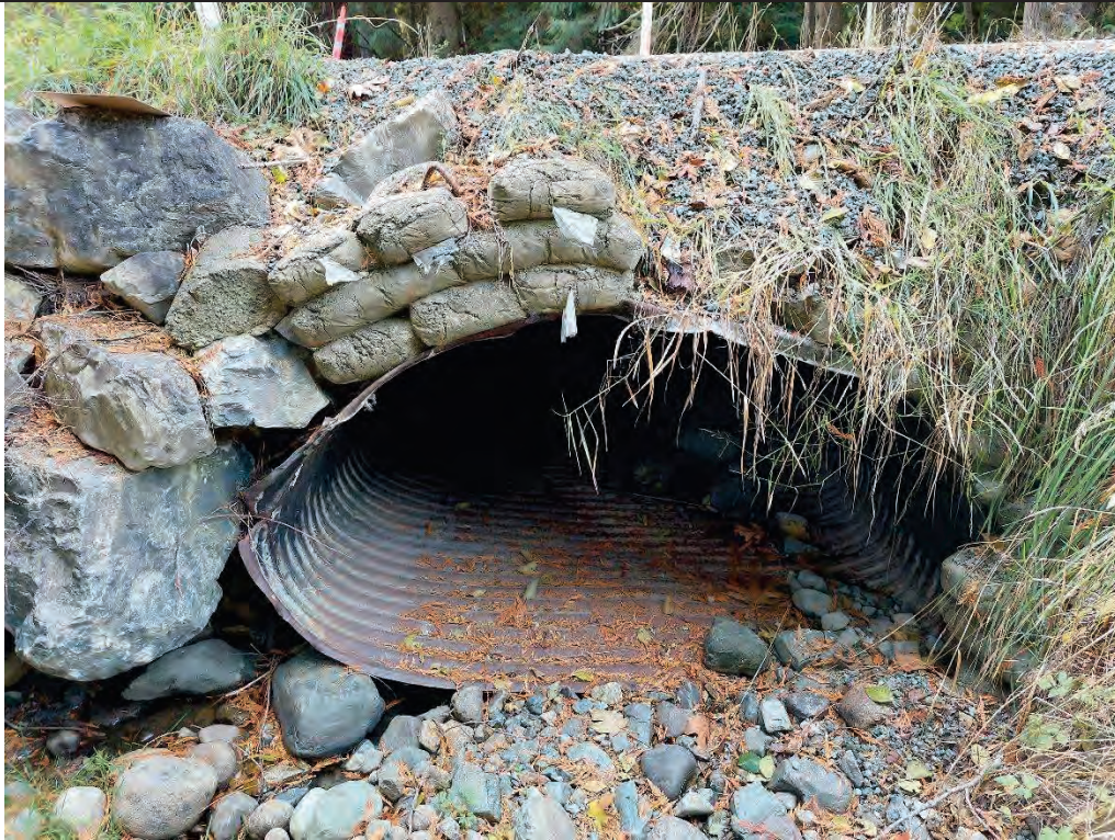
Culvert Inlet: Failed concrete bag headwall, culvert pipe visibly corroded, flow below gravel
