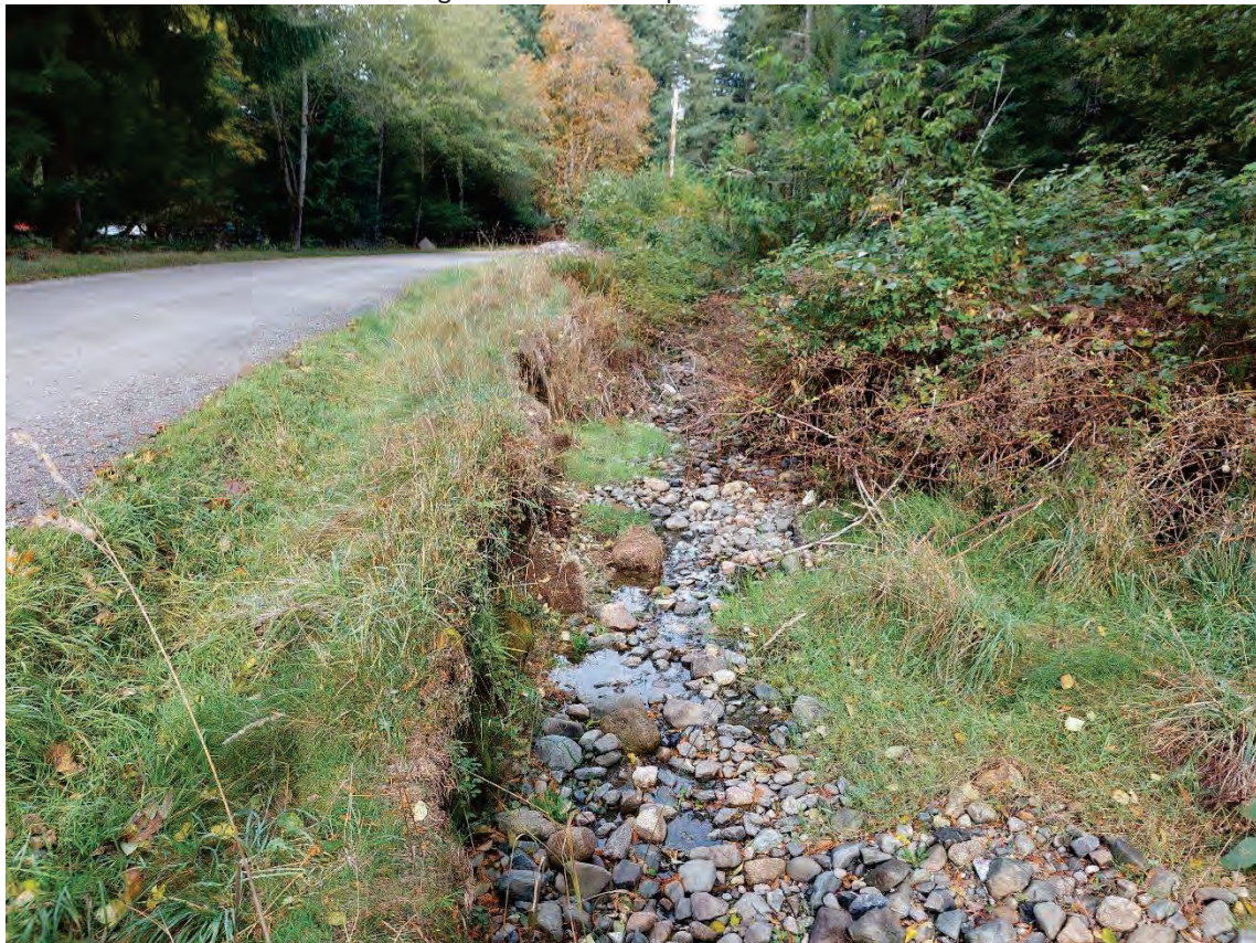
Upstream Channel at Bell Rd: Undermining of roadside ditch along 10m stretch
