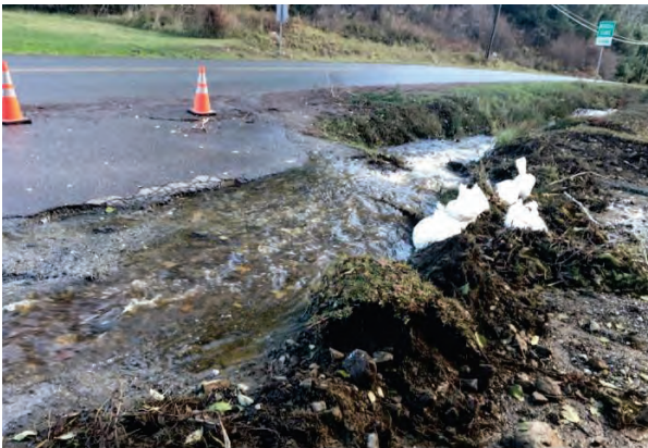
PHOTO 3: AREA 4 - OVERFLOW OF DRIVEWAY CULVERT (MOTI)
