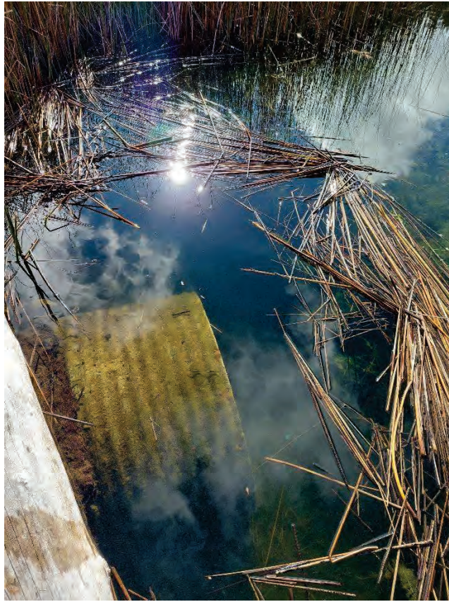
Culvert Inlet: Inlet fully submerged, log and reeds debris present above pipe
