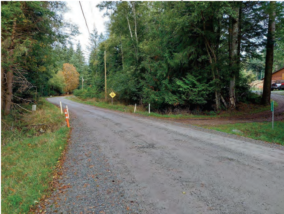
Bell Road above Staaf Creek: Gravel Road with eroding road embankment on the left side visible
