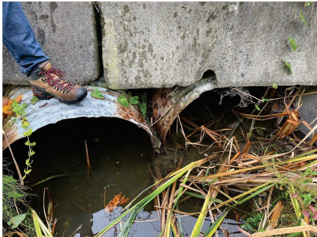
Culvert Outlet: Sediment Accumulation on right bank
