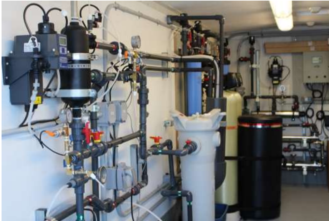
Figure 2.5 Filtration system in the pilot plant
